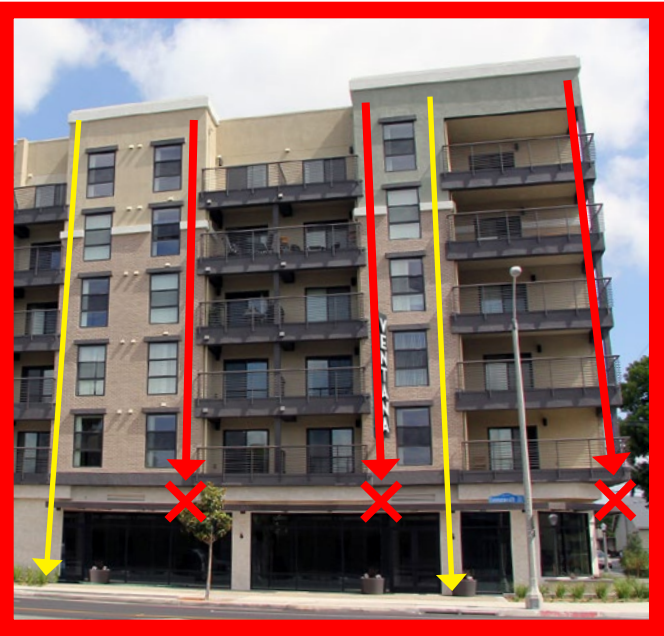
AVOID: Heavy upper floor building masses are not coherently supported. Vertical structure elements which frame upper floor bays randomly misalign with those in the building's base.
