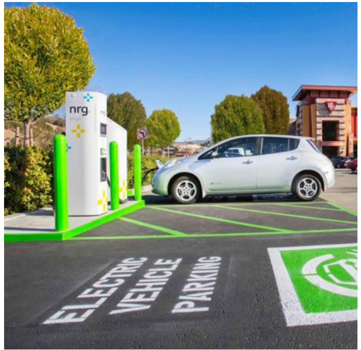
Example Electric Vehicle Charging Station.
